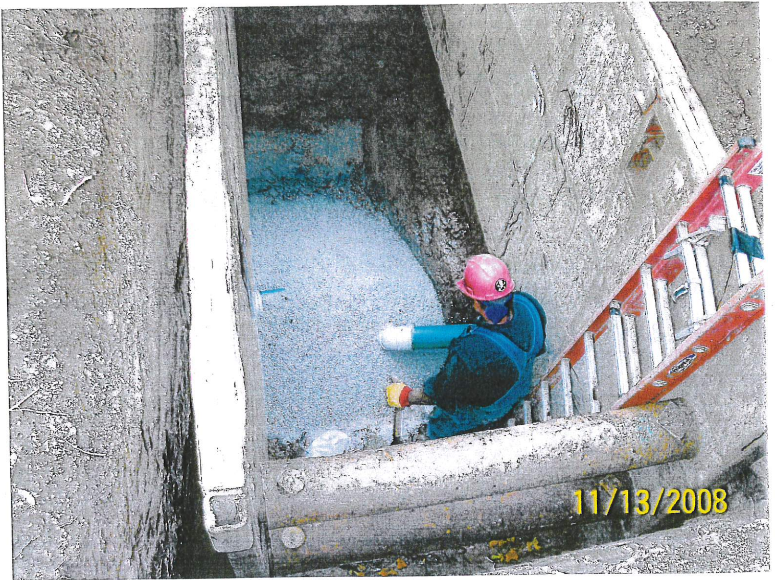
SPOT REPAIR AT STA 15+99 FOR 8108 N. NAVAJO ROAD AND 102 W. WILLOW ROAD
