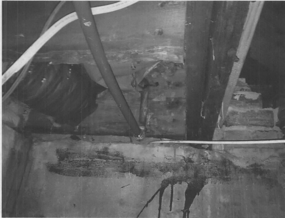
Photo 3 – Southwest corner – missing brick and joists turned 90 degrees unreinforced
