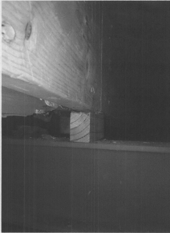
Photo 1 – Loose bearing block (note gap between block & joist)
